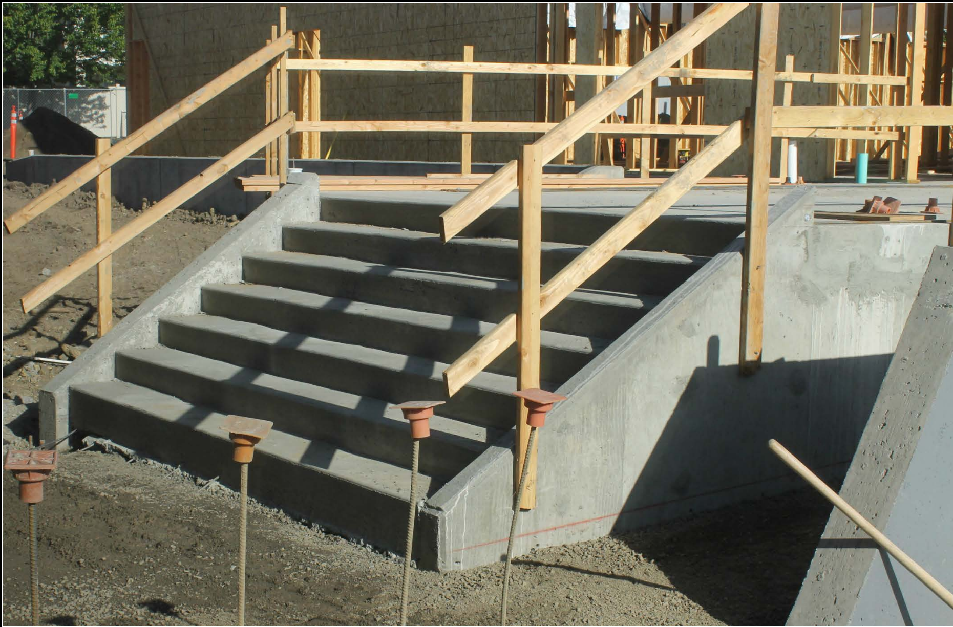
NEWSD 101 construction: Week 11 – May 28-June 1, 2018 Stairway & ramp connecting new & existing conference centers
